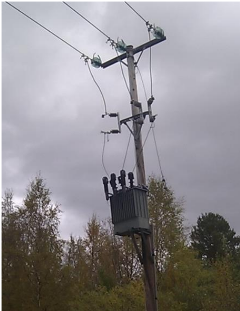
Transformator i stolpe.
